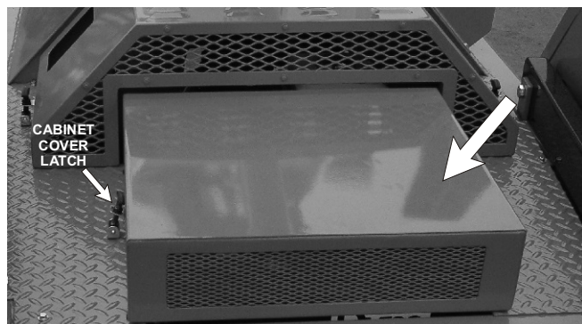
Figure 13.6 - DC Motor Battery Cabinet
